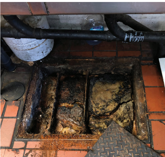
Example: Poorly maintained, and failing grease trap
